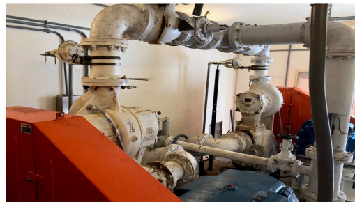
INDIAN HILLS SEWER PUMP STATION
